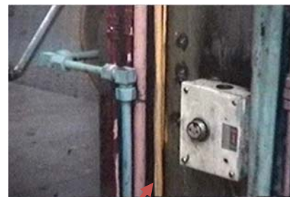
Liquid/ Lubrication Line
